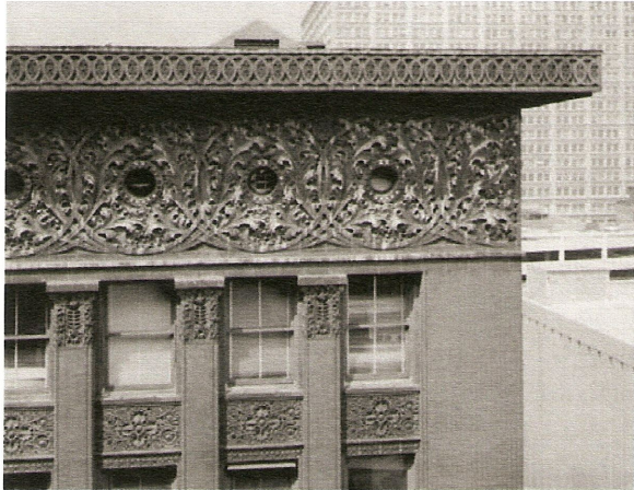
Ornamental cross pieces and the top port holes on the Wainwright Building
